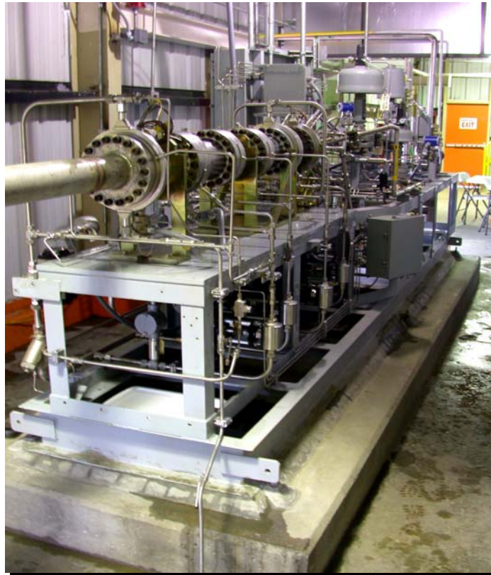
Fig. ES.2b. Fuel-Oxygen Combustor (Courtesy of Clean Energy Systems).
