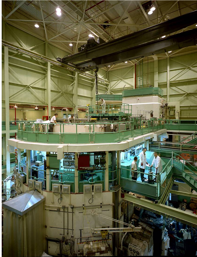
Fig. 47. The ORR inside its “confinement” building. (ORNL Photo 86784)
